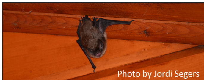
Figure 11. It may take more than one attempt to successfully exclude bats from a building.
